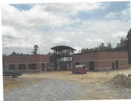
View of the construction of the back side of the Stead Center a few weeks ago. The SPPAHx office complex will be located here with its own separate outside entrance.
